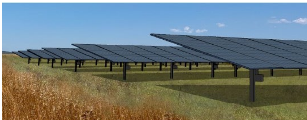
Rotello Solar power plants, Italy
