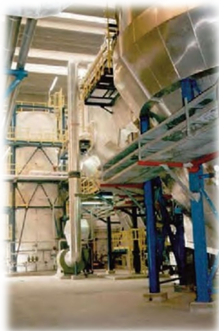
Busto Arsizio waste to energy plant
