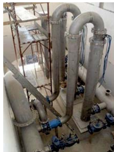
Detail of a pumping station
