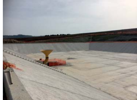
Detail of a basin
