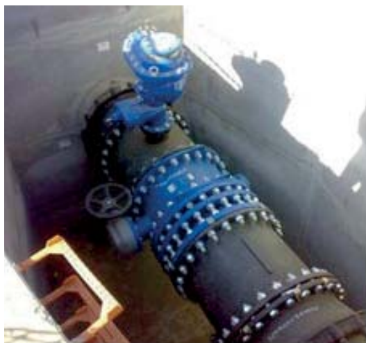
Detail of the main pipe
