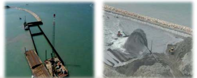
Construction phases of the refugee harbour: cofferdam sheet pile driving and reclamation filling
