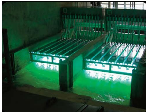
Savona wastewater treatment plant.
