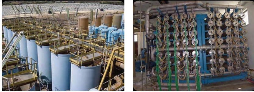
Priolo (Siracusa) drinking water treatment plant
