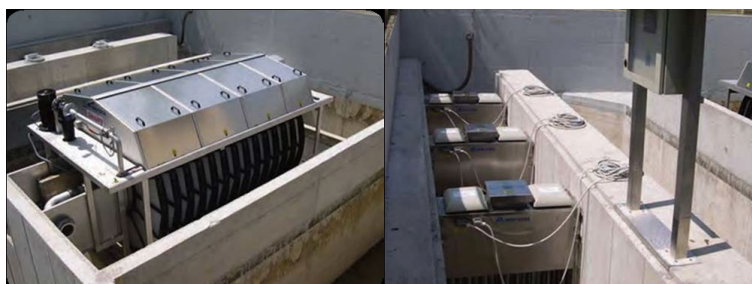
Castelfranco Veneto (Padua) wastewater treatment plant: filtration and disinfection plant
