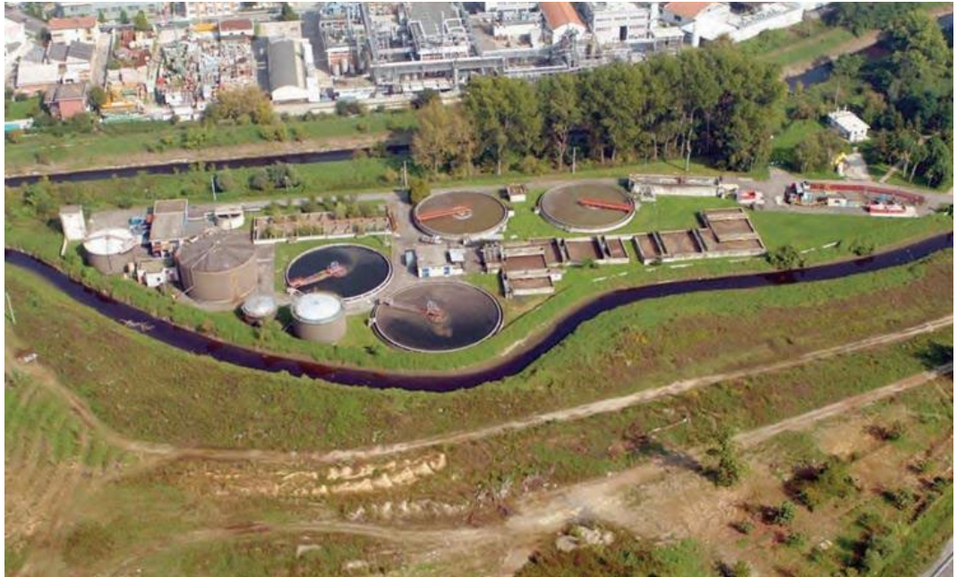
Rozzano (Milan) wastewater treatment plant
