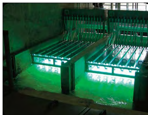
Savona wastewater treatment plant.
