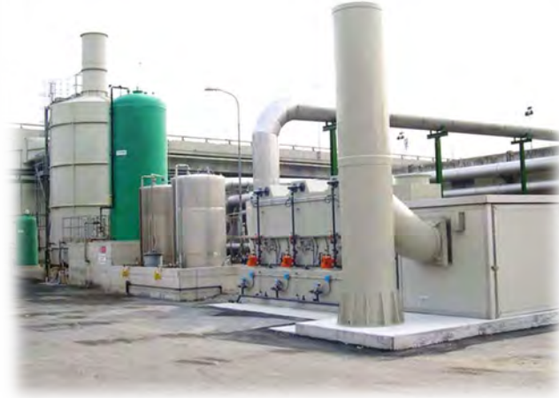
Finale Ligure (Savona) wastewater treatment plant: deodorization plant
