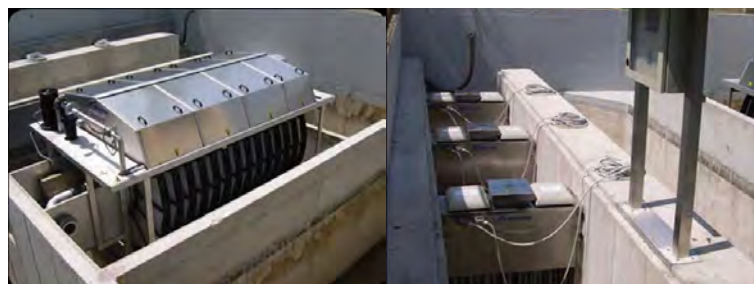
Castelfranco Veneto (Padua) wastewater treatment plant: filtration and disinfection plant
